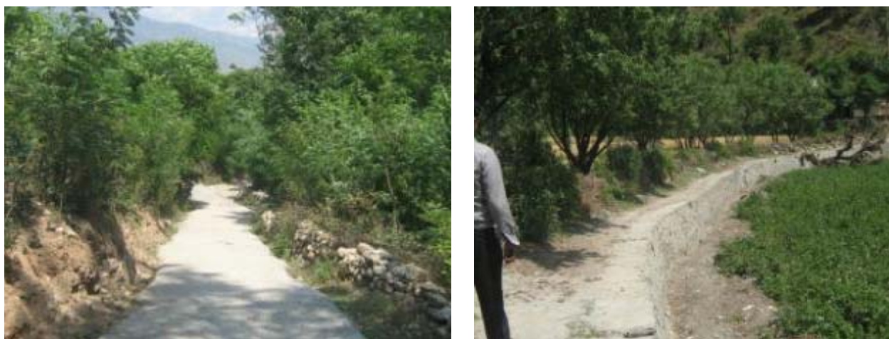
Photo 2.1 – An under construction Approach road and a Kuhl (irrigation channel) at Koyal village
