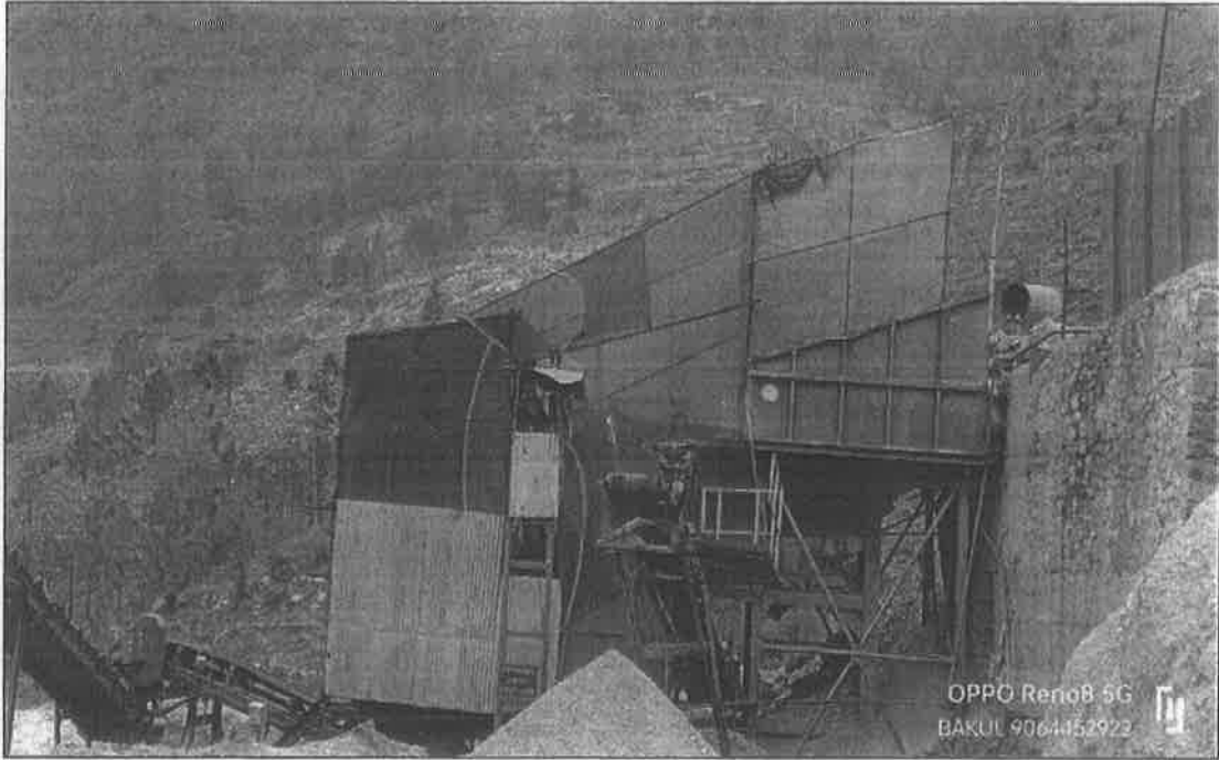
Picture-13. Crusher parts properly covered to prevent dust emission
