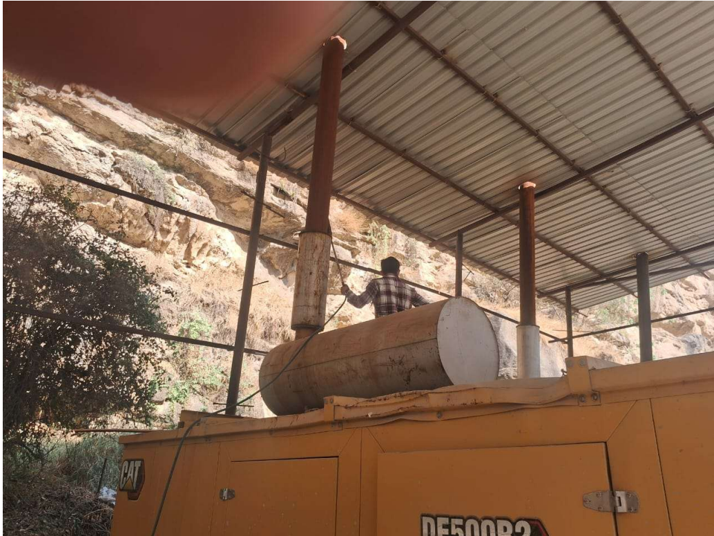
Comprehensive view of stack monitoring being executed on a large-capacity Caterpillar (CAT) Diesel Generator (DG) set. This physical verification confirms that the generator's integrated emission controls are operating efficiently and meet the standards prescribed under the Environment (Protection) Rules.
