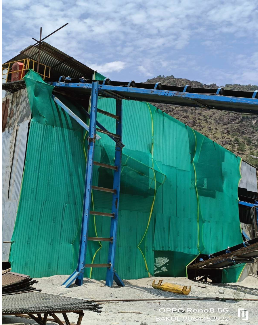
View of the stone crusher/aggregate processing unit completely enclosed with corrugated sheets and green dust-barrier netting to minimize fugitive dust emissions during operations.
