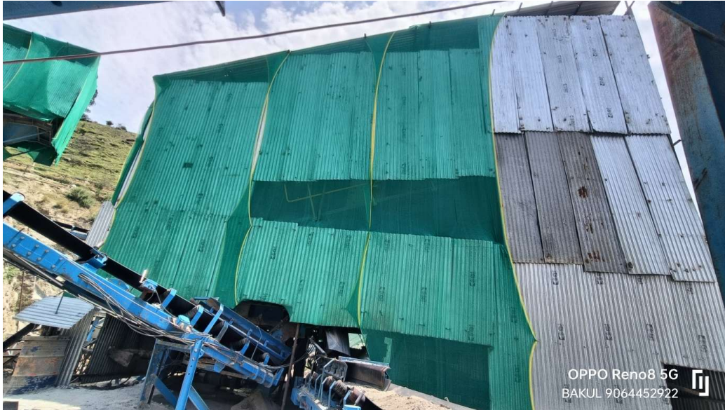
Detailed view of the material conveyor system protected by extensive wind-breaking dust screens, preventing wind-borne displacement of crushed aggregates.
